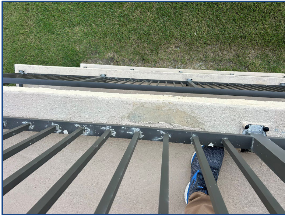
Photograph No. 41: Room 311 railings at the balcony.
