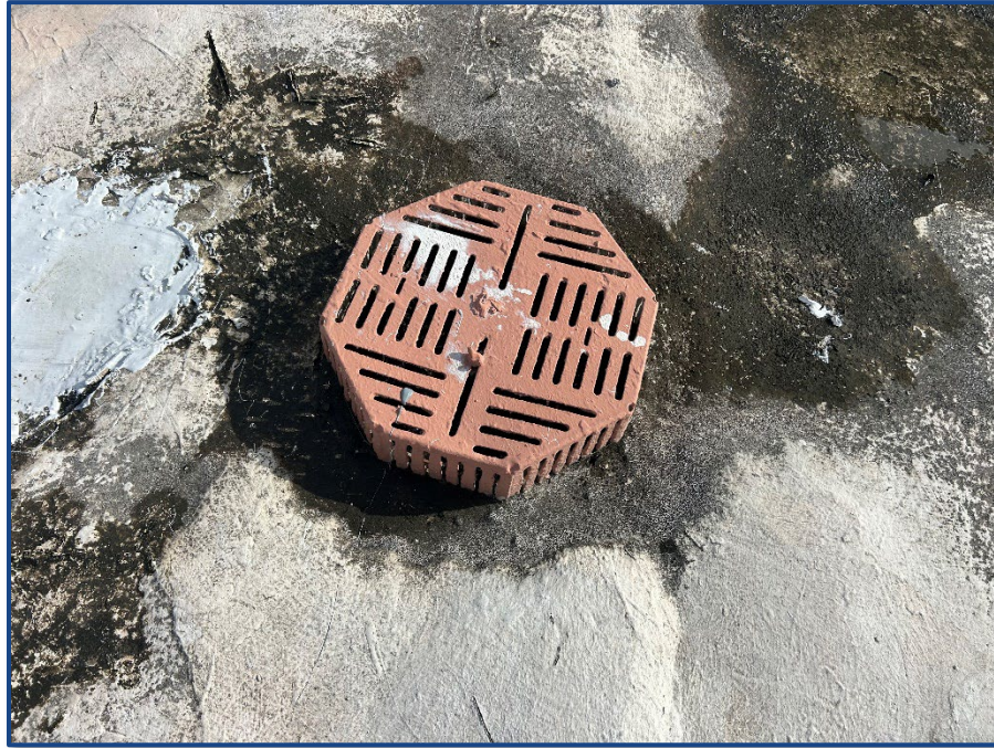
Photograph No. 17: Typical interior roof drain and cover in good overall condition.
