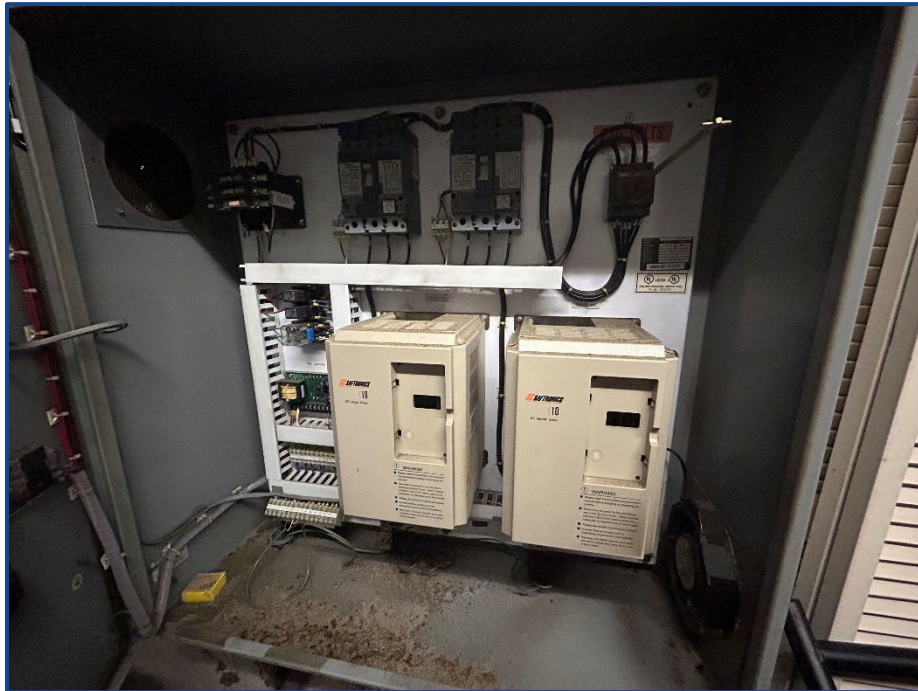
Photograph No. 23: AC industrial control panel.
