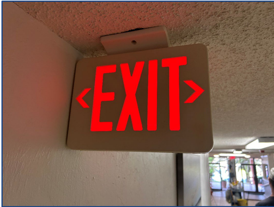
Photograph No. 35: Typical emergency exit sign in common hallway area.
