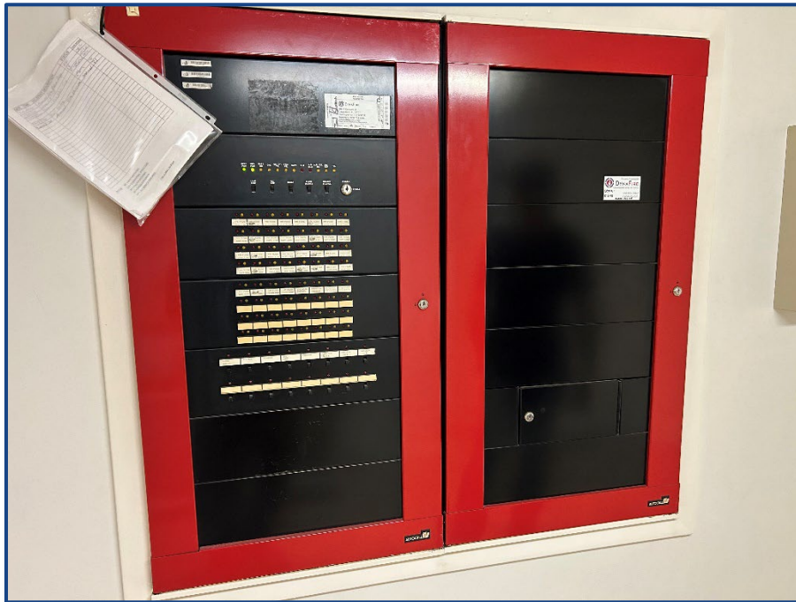
Photograph No. 18: Typical fire alarm control panel.
