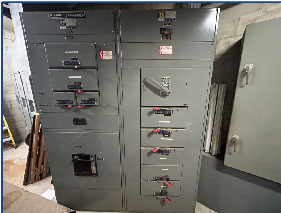
Photograph No. 22: Electrical power board with disconnect switches.
