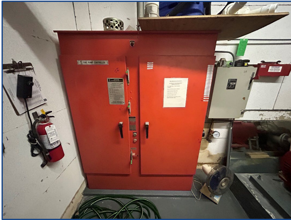
Photograph No. 19: Fire pump controller by Master Control Systems.
