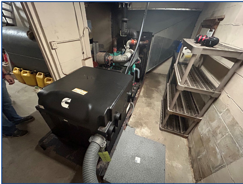
Photograph No. 24: Typical Cummins generator at garage floor utility room.
