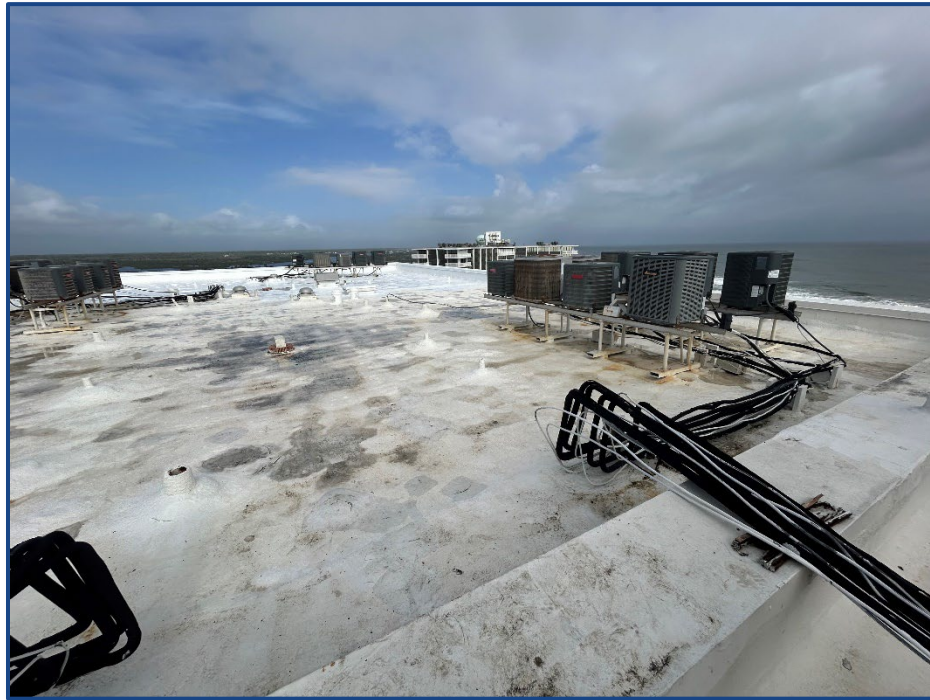
Photograph No. 15: Overall roof area at the north wing of the building.
