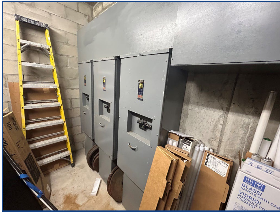
Photograph No. 21: Typical electrical main service panels.
