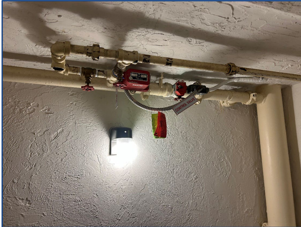
Photograph No. 32: Typical lighting and fire line in the interior stairwell.
