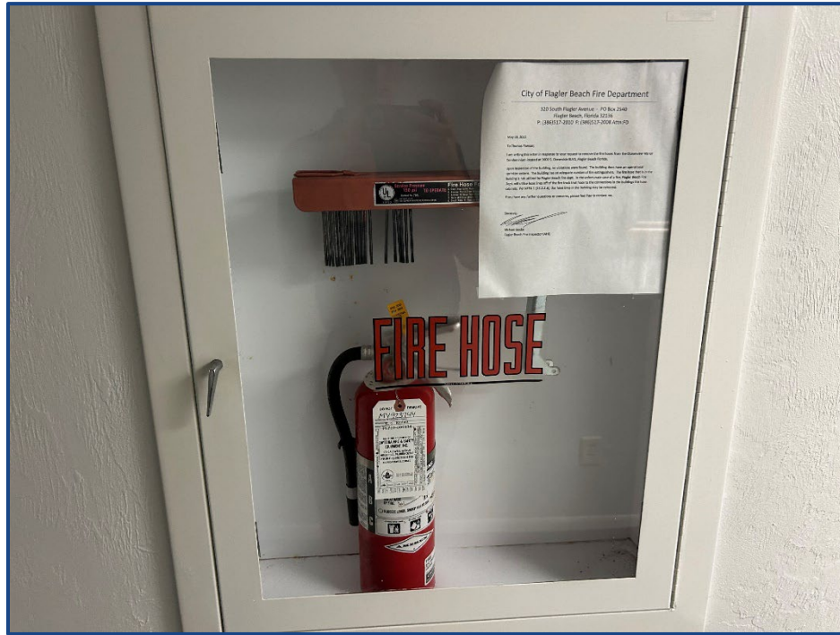
Photograph No. 31: Old fire hose access standpipe out of commission and fire extinguisher.
