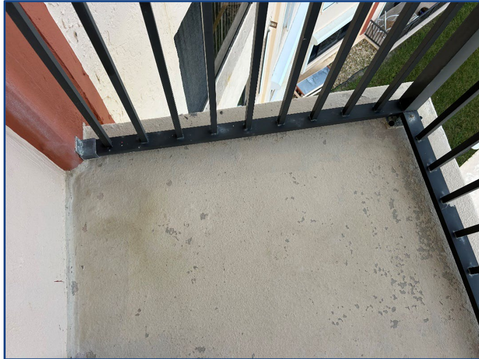
Photograph No. 46: Room 513 balcony with aluminum railings and some chipped paint.
