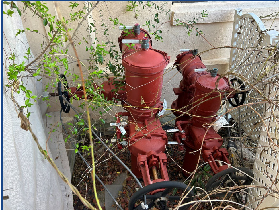
Photograph No. 38: Typical backflow at the west building perimeter.
